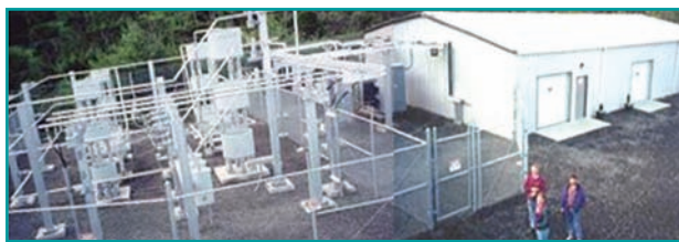
figure 5. GE/GNB and Metlatkla Power and Light battery energy storage system in Alaska. (Reprinted with permission from George Hunt, GNB/Exide.)
